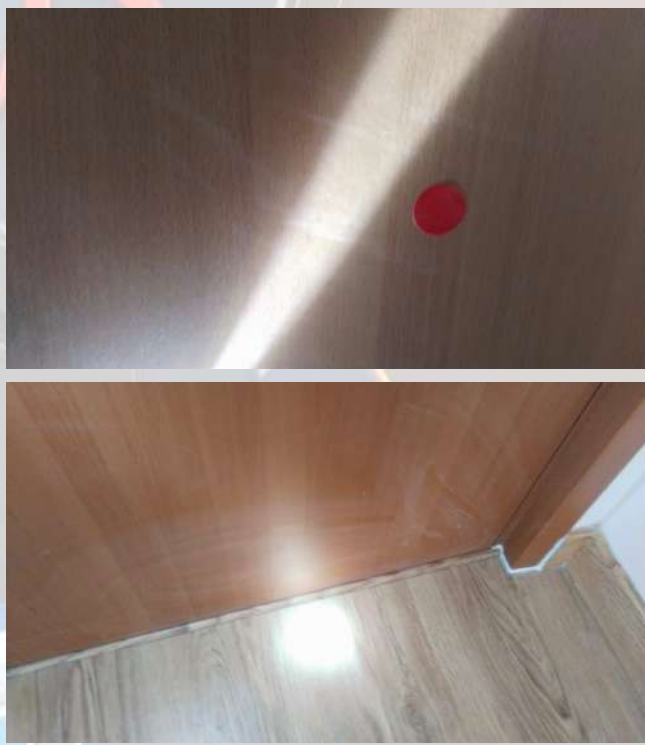
Paint stains makes found on door front and back portion
