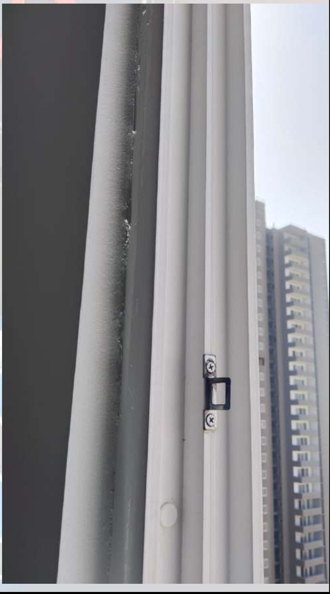
Window frame packing finishing not proper , proper finishing required .
