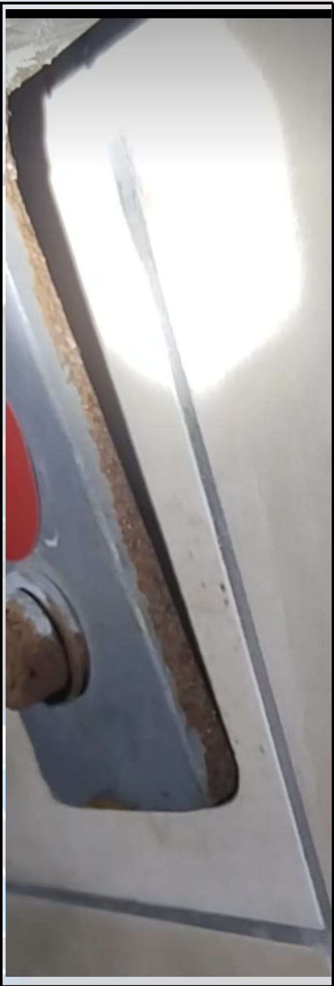
Granite slab metal holder and nut bolt started getting rusty , painting required
