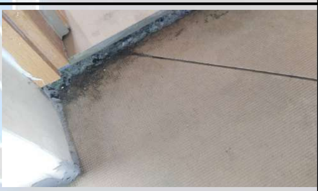
Door entrance tile grouting not done from the passage side
