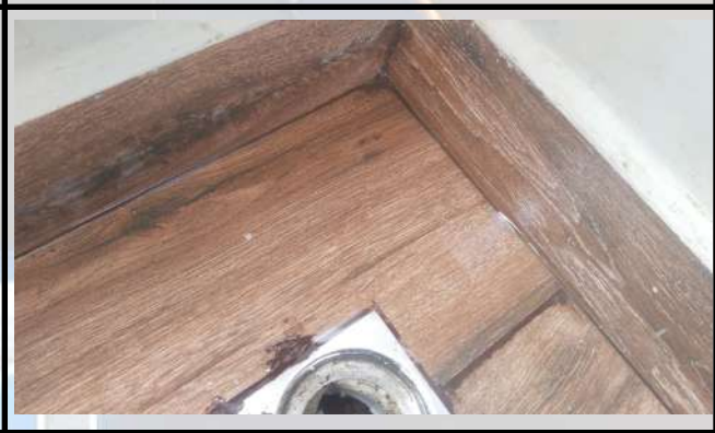
Water accumulates near the drainage pipe left corner .
