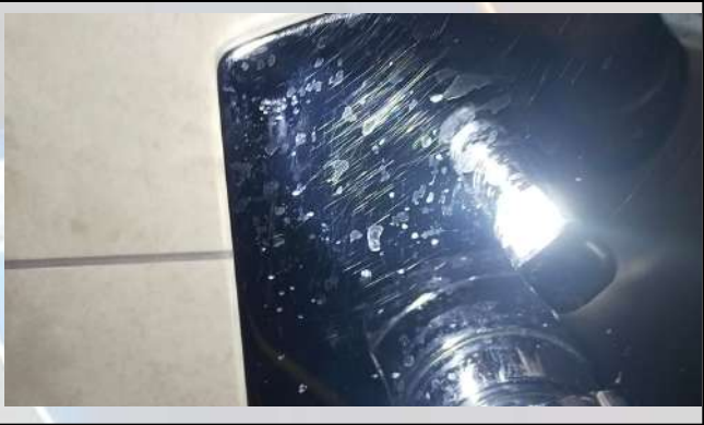
Scratch marks found on wall mixer tap
